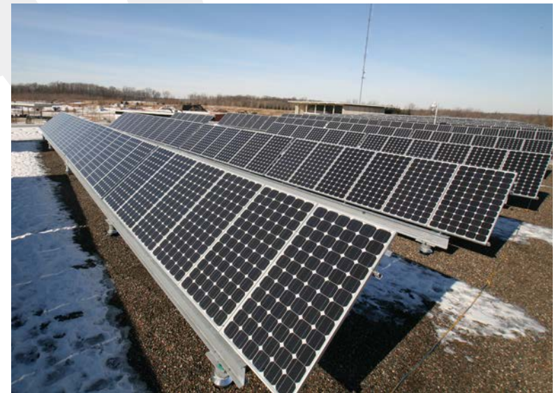
Solar panels on the roof of Hennepin County Public Works Facility in Medina.
