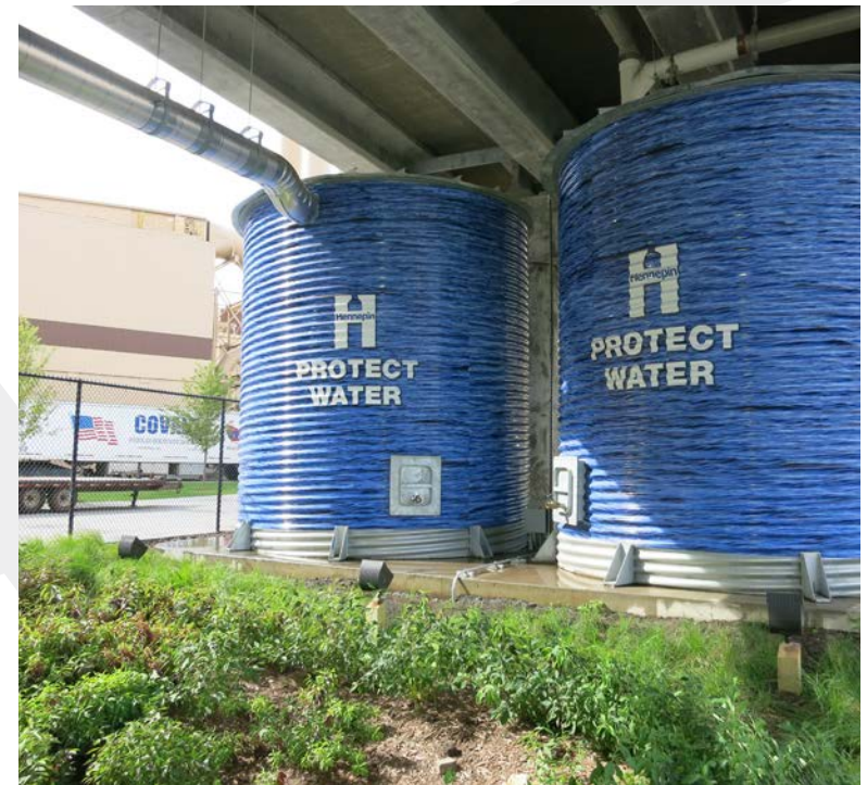
Target Field Station includes a variety of features, including these cisterns and bio swale that capture and filter approximately three million gallons of rainwater and snow annually.
