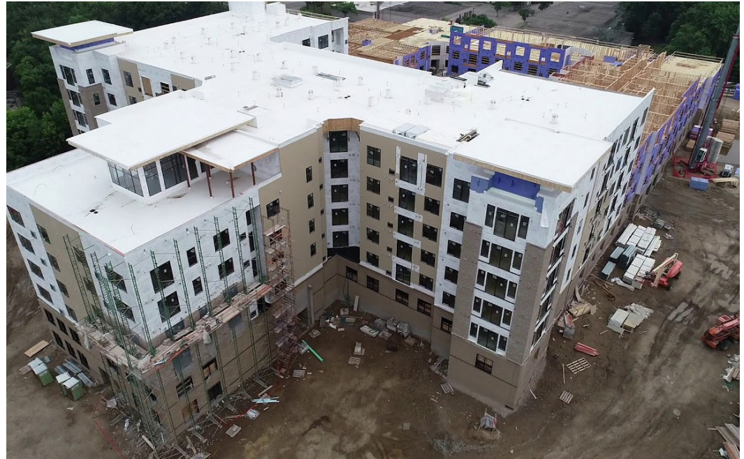
Construction at RiZe at Opus Park Apartments along the Southwest LRT line in Minnetonka.
