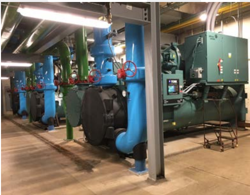
Capital project in 2017 to replace electric chillers at the Hennepin County Energy Center with more efficient models, saving $175,000 per year in electricity costs.
